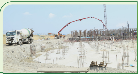
The work is in progress against facilities to M/S. TCCL- Frame JV, a joint venture lead by Toma Construction Limited.
