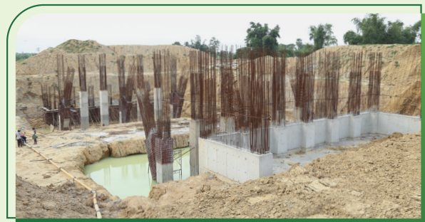
The work is in progress against facilities to Western Engineering Limited for completing different Government construction works.
